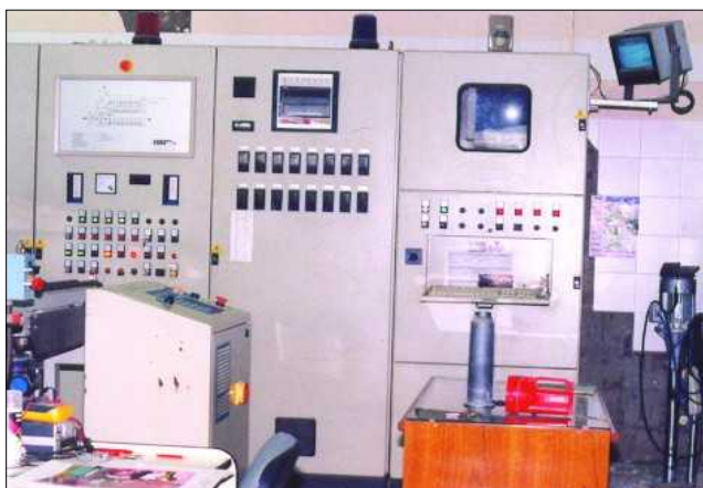
Paneles de control
